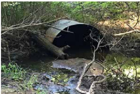
The existing 54-inch by 72-inch CSP arch culverts at the park roadways were severely deteriorated and undersized, causing fish passage issues, erosion, and increased velocities in the stream.
